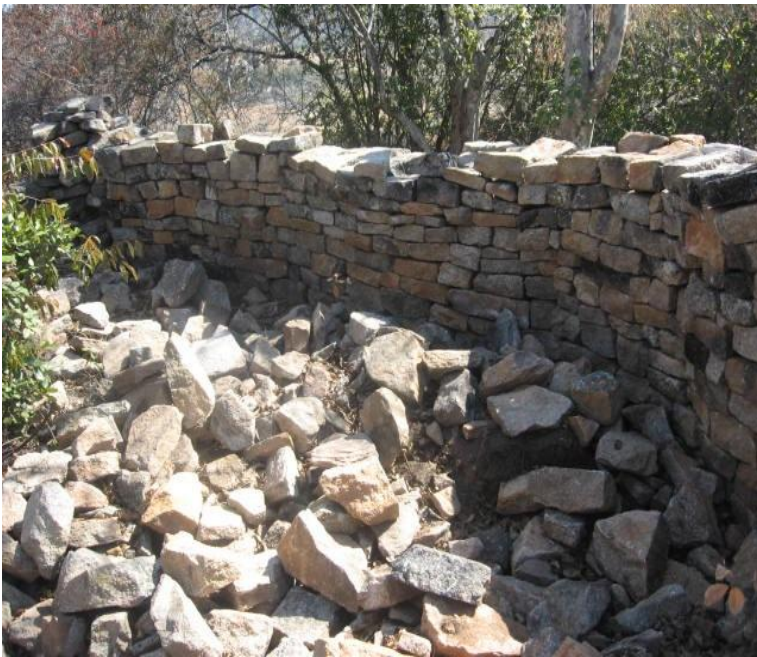
Fig 8: After vandalism (Source: restoration Report, E4 File)
